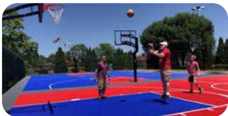
Complete renovation of outdoor basketball courts and hoops, tennis courts and addition of pickleball courts
